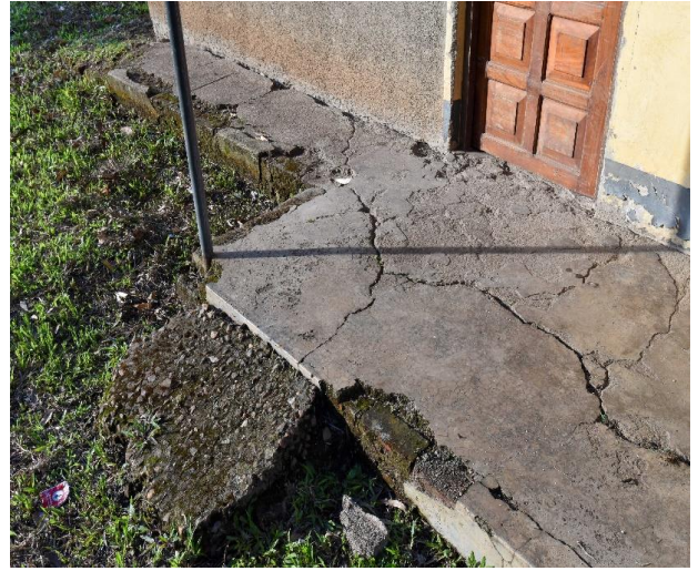
Cracks discovered at Katerera Beat
