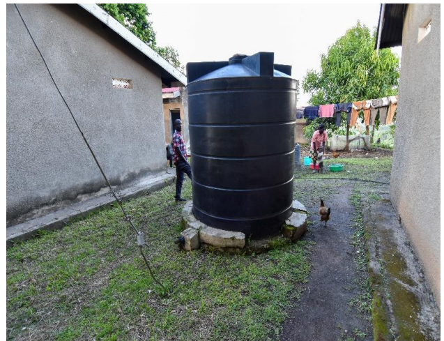
Cracked Tank base at Katerera
