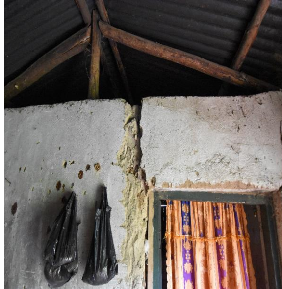
Structural cracks in walls at Bihanga station
